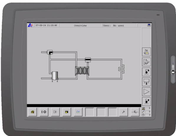
Figure 11. An overview picture of the PLC operator panel.
