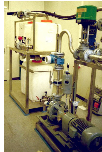
Figure 22: Test bed: Commissioning phase
